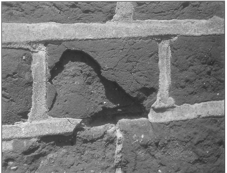
The danger of using cement-rich mortars: frost damage caused to a soft red brick. Moisture, unable to escape from the impermeable mortar, has frozen, causing the brick to spall.
