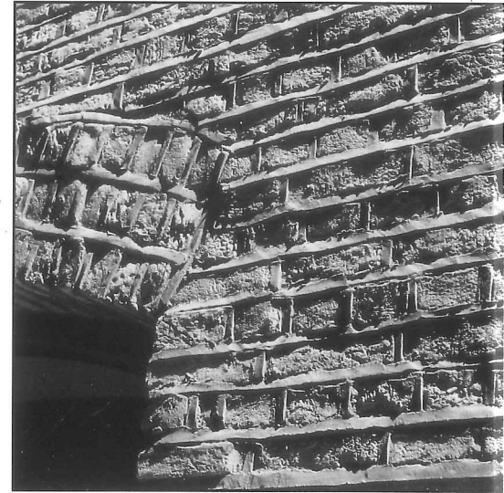
This Victorian building has suffered both from harsh cleaning and unsympathetic repointing. The former has eroded the surface of the bricks, creating a pitted, irregular effect which is emphasised by the thick strips of unsuitable, cement-rich ribbon pointing.
