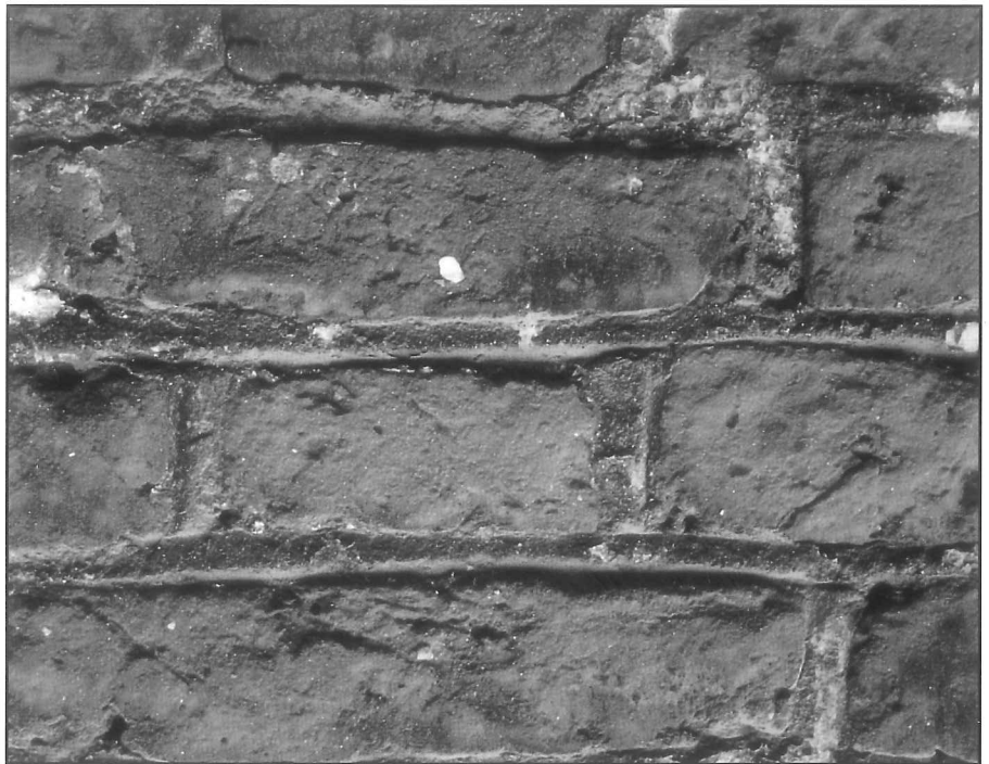
Detail of a brick wall at Hampton Court, dating from the 1530s. Note the thin and irregular shape of the bricks. A double-struck joint finish of lime mortar has miraculously survived in crisp condition. Every effort should be made to discover the original joint finish of a wall and to replicate it using a lime-based mortar.
