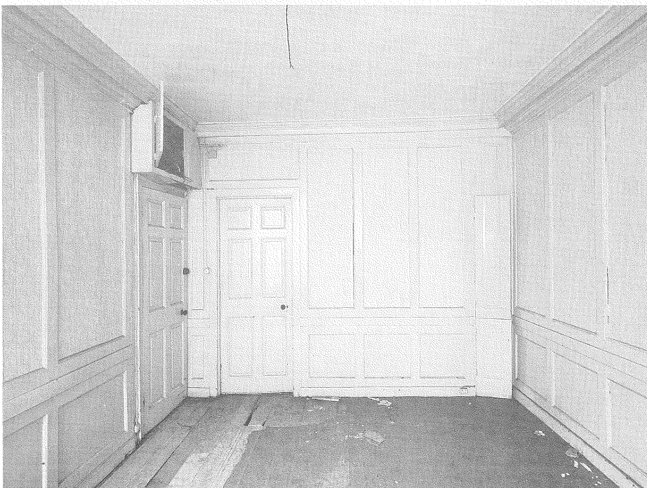
31 Great James Street; simple panelling, a Tuscan cornice, and raised and fielded panels on the door
