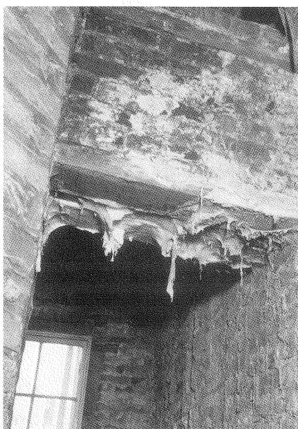
Non-destructive techniques should be used to eradicate dry rot. Adequate ventilation is essential
