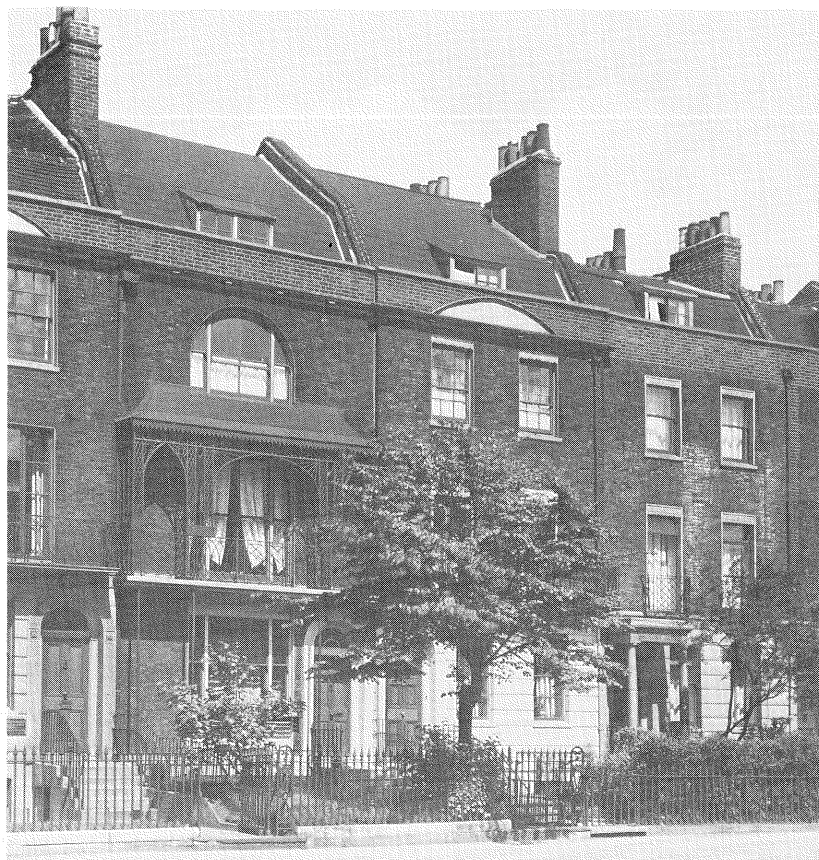
Mansard roofs have two slopes on each side, the lower face being more steeply pitched than the upper, thus providing more space for accommodation than would be possible with a conventional roof of single slope
