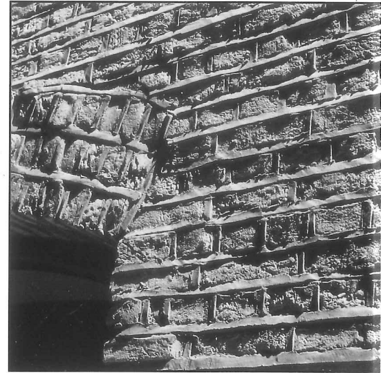
This Victorian building has suffered both from harsh cleaning and unsympathetic repointing. The former has eroded the surface of the bricks, creating a pitted, irregular effect which is emphasised by the thick strips of unsuitable, cement-rich ribbon pointing.
