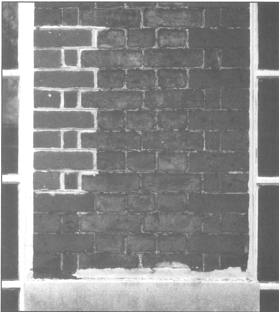
Ill-considered partial pointing often has an adverse visual effect on brickwork. This early eighteenth-century example shows two areas of repair which damage the appearance of this pier. The area on the left has correctly reinstated the penny-struck finish, but the lime putty has been smeared over the arrisses so that the joints look too prominent. The repair at the bottom of the pier has greatly widened the mortar joint and ruins the distinction between the brick pier and the stone plinth.
