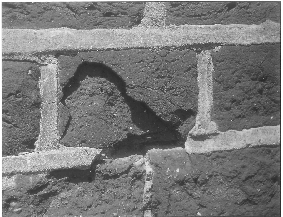
The danger of using cement-rich mortars: frost damage caused to a soft red brick. Moisture, unable to escape from the impermeable mortar, has frozen, causing the brick to spall.
