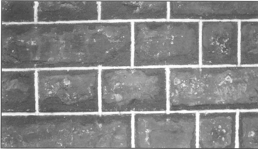
Tuck pointing: a recent London example, showing the neat strips of lime putty set into wider mortar joints to create the impression of crisp new work upon an extensively repaired wall.
