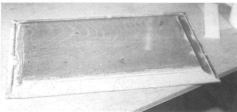
Panelled door in course of upgrading with intumescent membrane. The lower image shows a removed panel with intumescent membrane applied to the front edge only.
